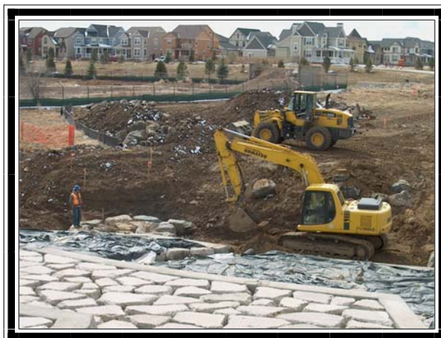
Westerly Creek North is an 8-month erosion control project within the Stapleton Redevelopment Project. At press time this project is near completion. Territory Unlimited brings Staplestone from RMCI's stockpiles on 56th Avenue.
