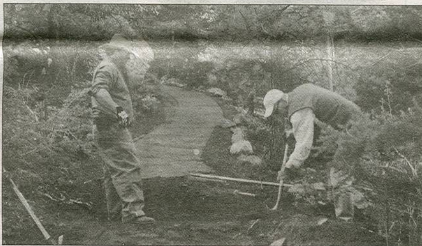
CCA Associate Council Chairperson Mark Lillemon and CCA staff member Brian Garber construct a water bar in a trail to create proper drainage.
